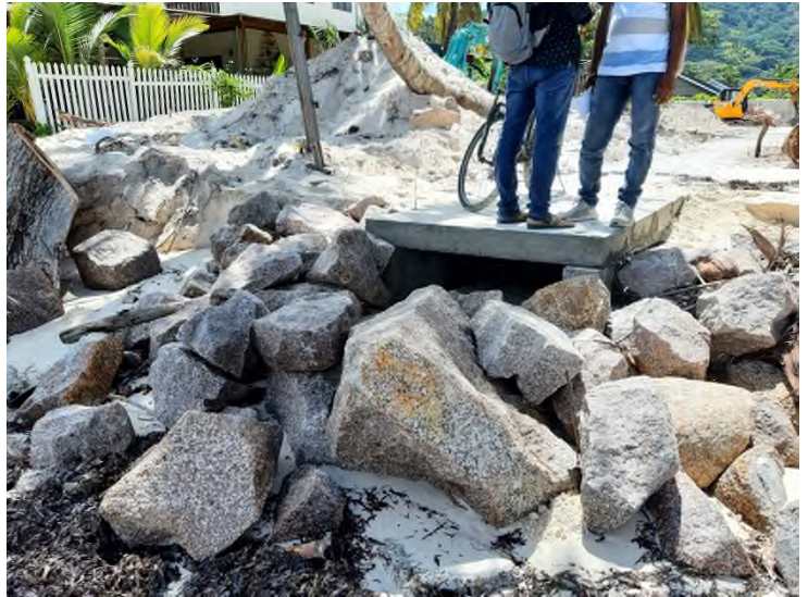
Rock filter at drain outlet.
